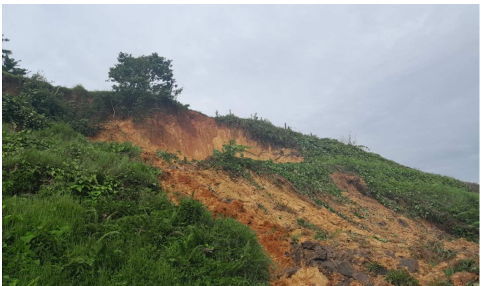
Figure 12l: Landslip on Kings Road at Viwa, past Korovou on the 25 th . Source: Fiji Roads Authority
